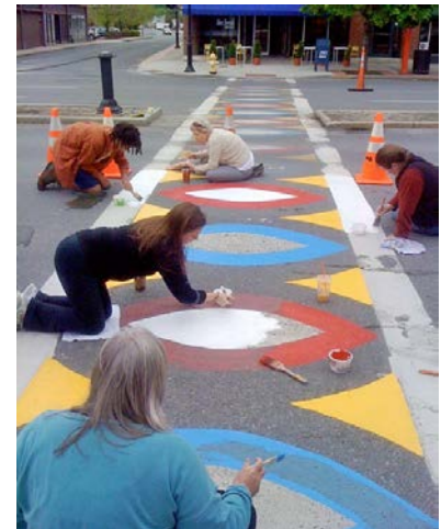
Creative crosswalk designs are possible and can help remind motorists of a special crossing area like at a school.
