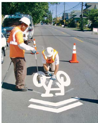
A sharrow, or shared lane marking, being installed. Sharrows indicate to bicyclists the best place to ride in a lane shared with vehicles and remind motorists to expect and share the lane with bicyclists.
