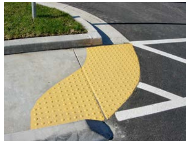
Brightly colored tactile materials highlight the edge between sidewalk and street for people with a range of vision impairments.
